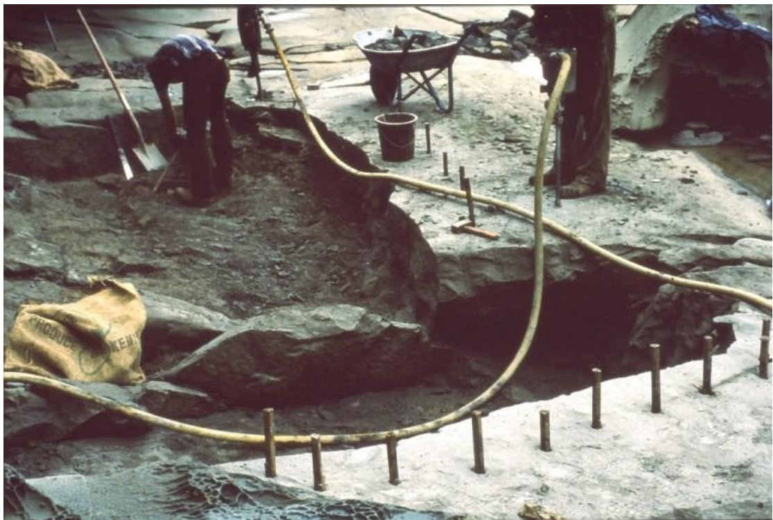
The start of Lake Copco site, using plugs and feathers to break the rock. Courtesy of T.H. Rich Collection.
